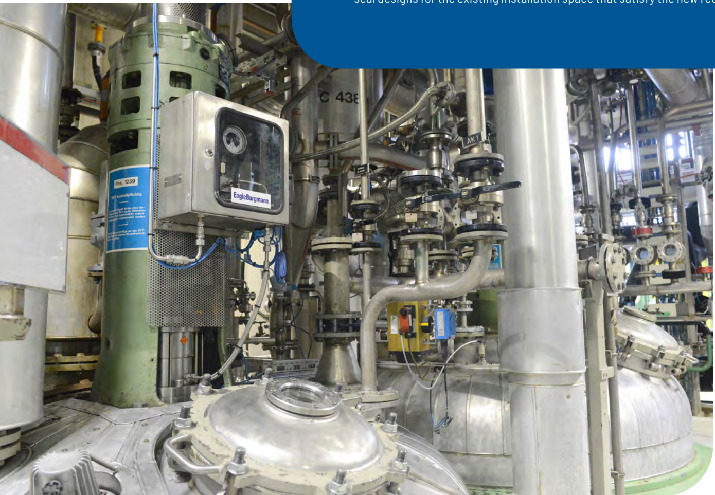
The upper parts of two containers. The SeccoMix can be seen on the left through the bottom opening in the green shaft housing. On the top are the instruments for the supply system for the seal.
