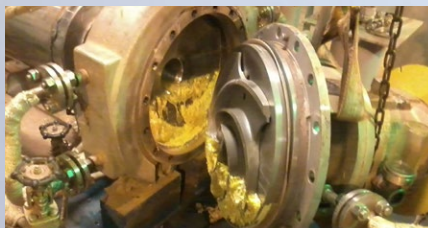
Examples of crystalline sulfur leakage outside and inside of pumps
